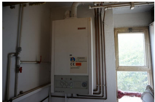
Piano seminterrato – Caldaia
